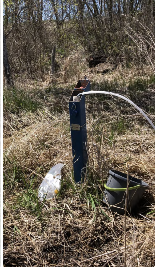
Photo 25: view of monitoring well MW107.
