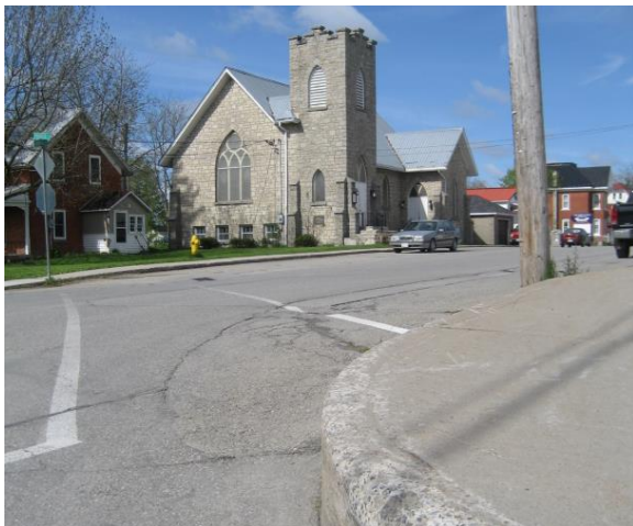
Reduce tall curbs during future reconstruction to improve crosswalk accessibility for users of mobility aids
