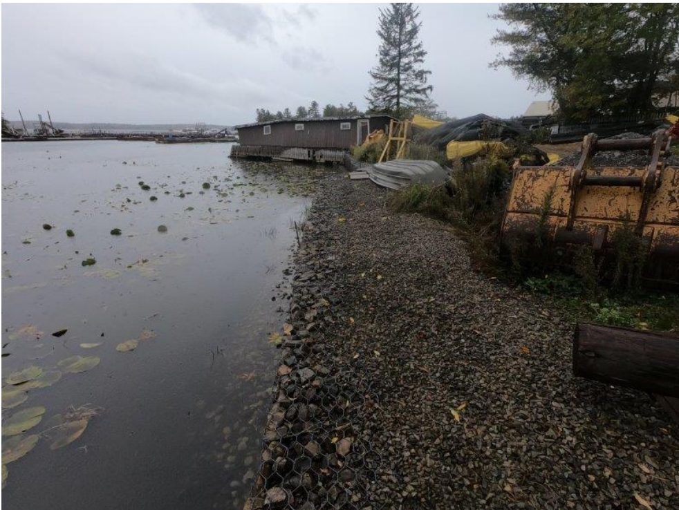
Photo A6: Looking Southwest along shoreline towards boathouse, North end of gabion wall section (2022)
